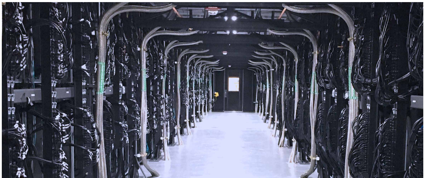
A close-coupled, evaporative cooled, Gen 3B data center hot aisle with 60U racks with up to 280 disaggregated servers/rack and up to 43 kW/rack.
